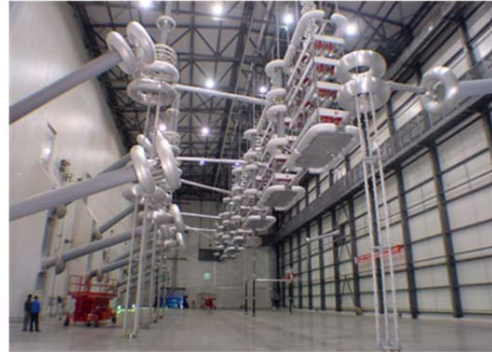
Figure 5: Example of a HVDC (inside of converter hall)
